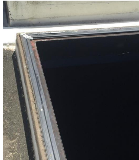
Ventilation unit rubber seals
