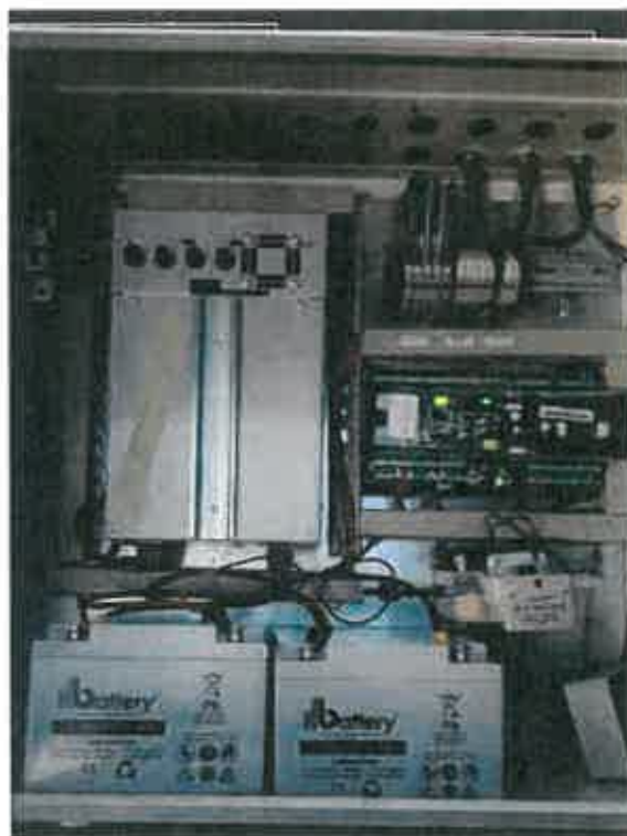
Fig 3 – Power Supply Unit
