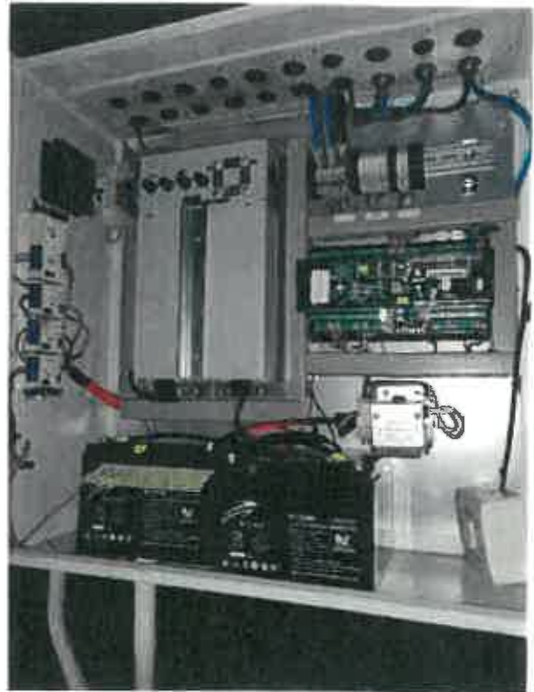
Fig 2 – OS2 Control Panel
