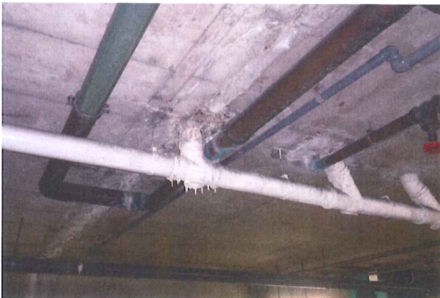
Cracks and joints that need to be sealed
