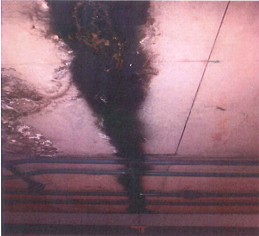
Crack in service tunnel
