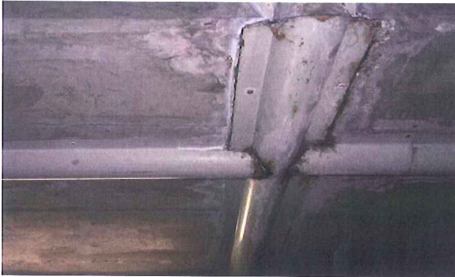
Expansion joints that need to be sealed
